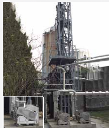
• Biogas plant: ROBOX evolution BIOGAS blower unit
