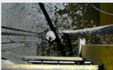
Warman® SHW pump in the event pond application.
