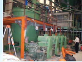
Pump's inspection Service
