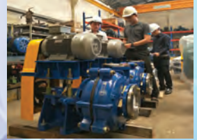
Pump's installation service
