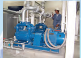
Site test & commissioning service
