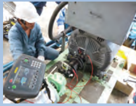
Shaft alignment service
