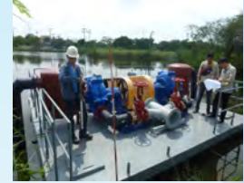
Site test & commissioning service
