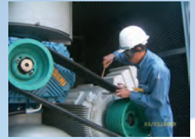
Belts tensioning set up
