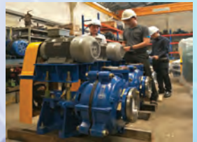
Pump's installation service
