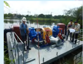
Site test & commissioning service
