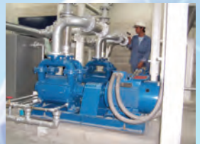
Site test & commissioning service
